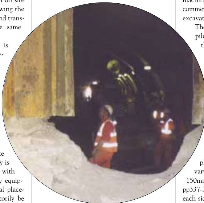
Unusual view through the base of sheet piles at the end of the tunnel excavation
