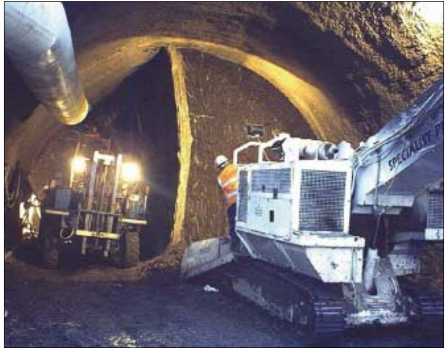
Tunnel construction showing the side drift technique with special access equipment for support installation (left) and the Schaeff excavator from Specialist Plant (right)
