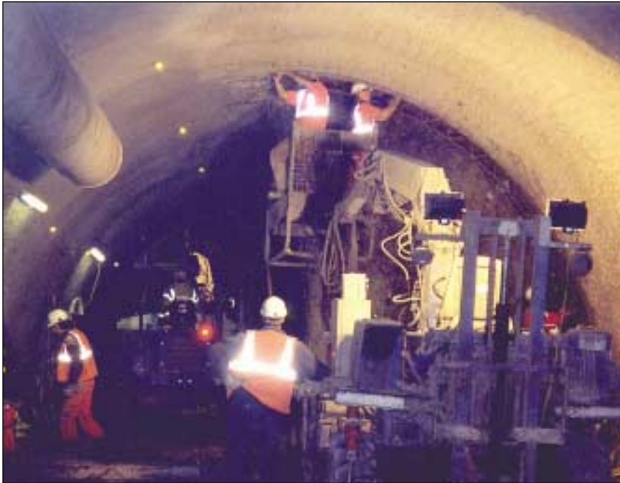
Erecting the lattice arches and wire mesh prior to shotcreting using specially made access equipment
