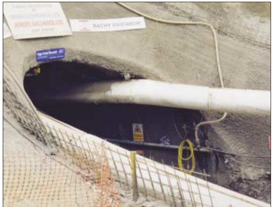
The tunnel portal with shotcreting complete on a reinforced structure with soil nails
